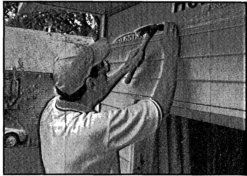
Lee French, Habitat for Humanity volunteer, installs siding on the Habitat for Humanity home this past Saturday.
